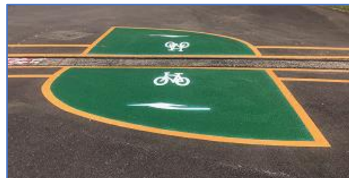
Painted guidance for crossing the tracks at Newington Armory. Photo by Charlene Bordley.
