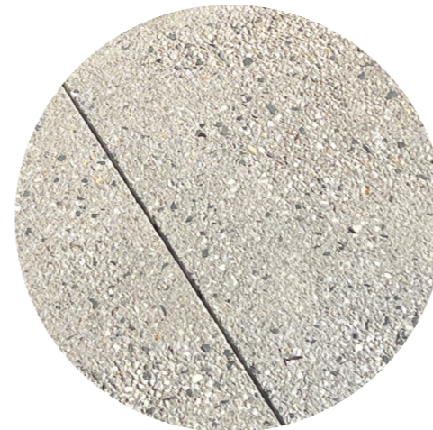
Field Level Paving / Internal Floor Washed Aggregate Concrete slab with sealer. Slip Rated and able to be hosed down
