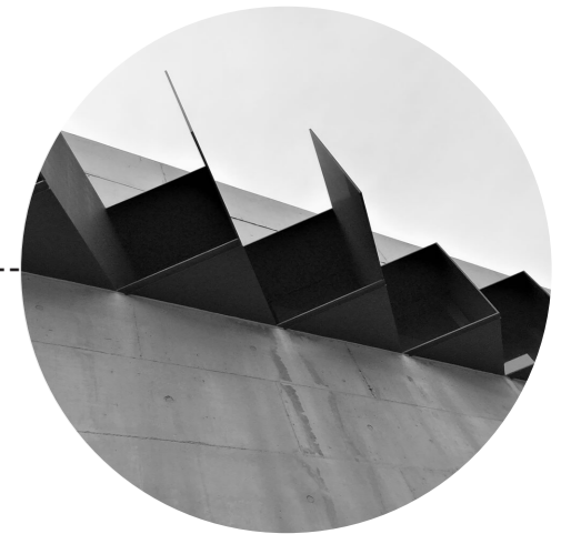
Steel Plate sunshading
