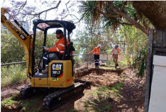
Figure 21. Overview of TT1 location, looking northeast. Note the confined space and fence constraints that moved the proposed location further west and changed orientation.
