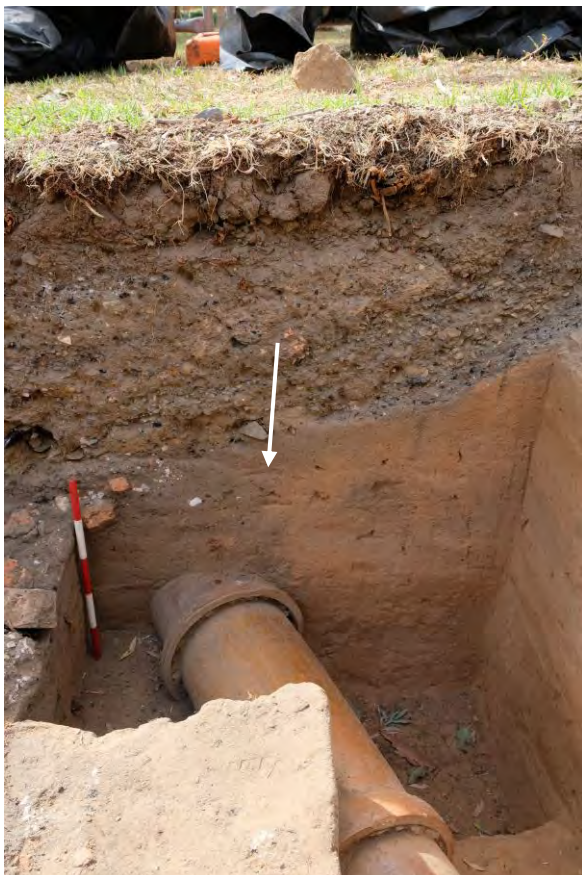
Figure 24. Section of ATP5 North with eastern extent of collared pipe (pipe cut and fill marked). Also showing large landscaping cut truncating the PSB, facing east.
