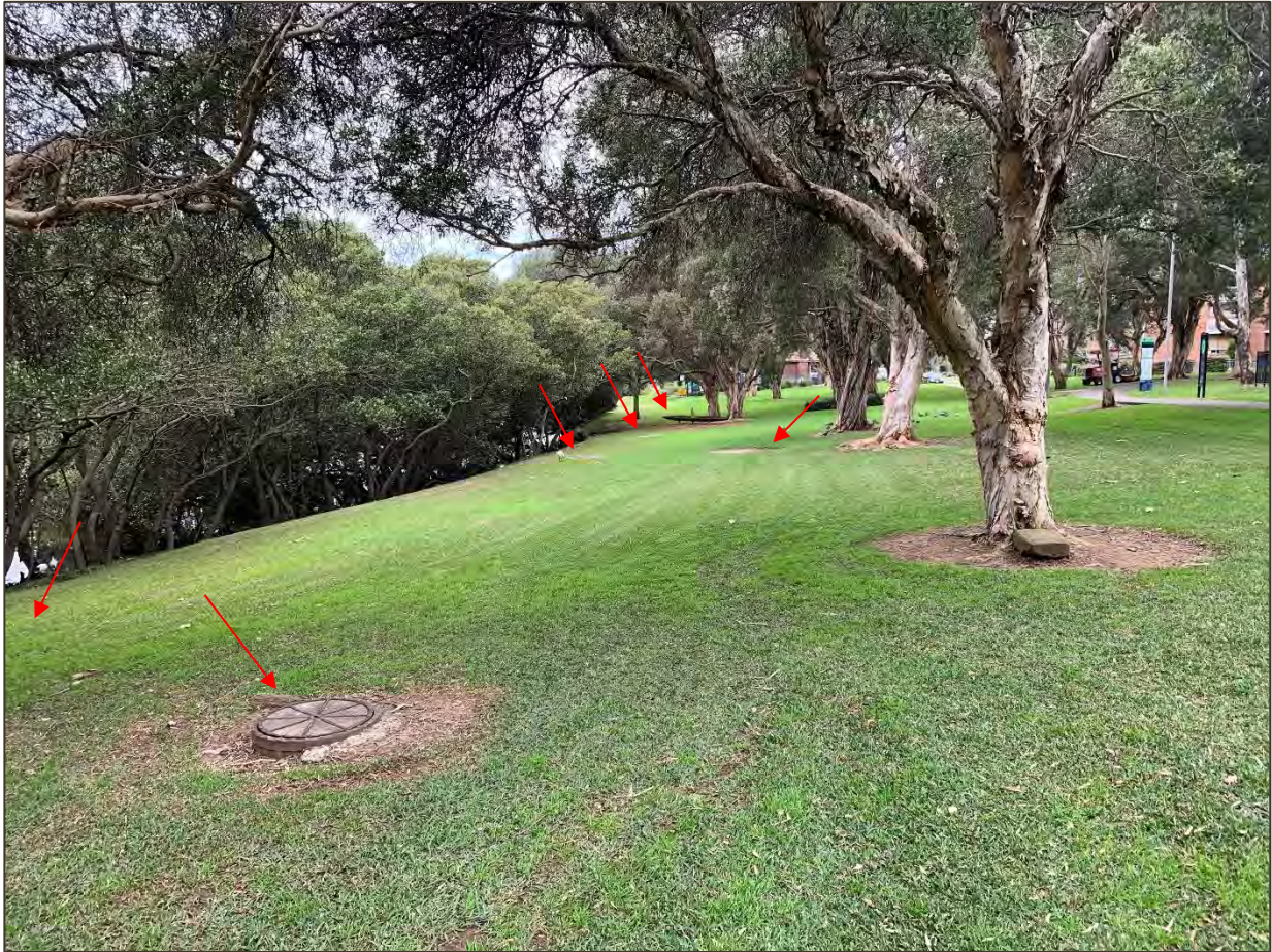
Figure 40 Disturbance associated with services. Manholes/inspection pits marked with red allow demonstrating a portion of the feature’s extent.
