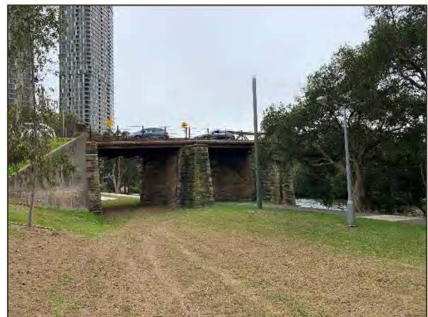
Figure 12. Disturbance associated with Gasworks Bridge.
