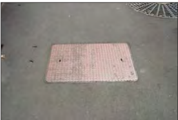
Steel pit cover
