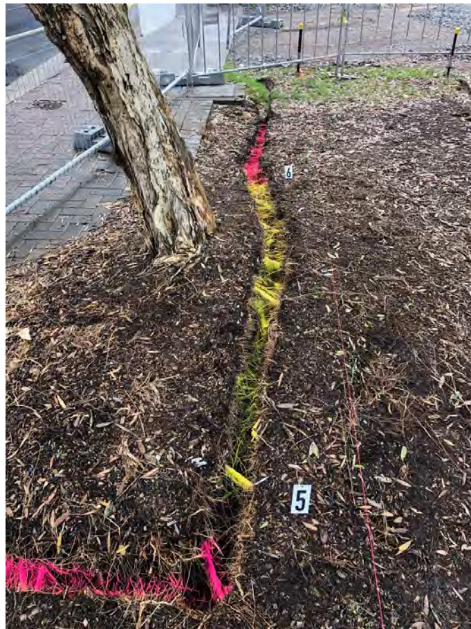
Plate 10: Example of Hydro excavation and the extent of roots that can sometimes be encountered. P. Vezgoff.
