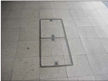
Paving infill lid in unit pavement
