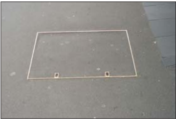
Paving infill lid in asphalt
