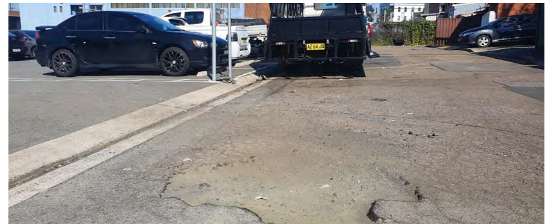
Condition of Cowper St laneway.
