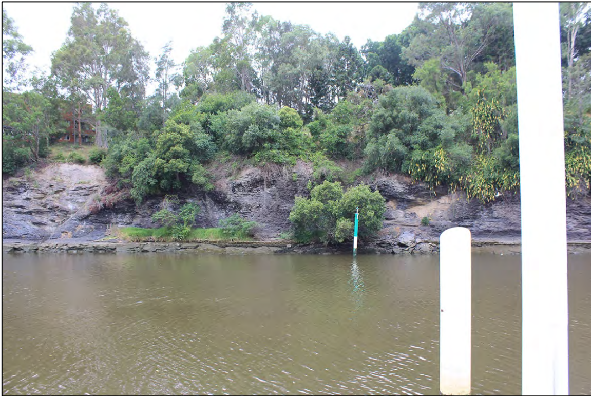
Figure 4.4: View of the opposing bank showing the exposed shale and minimal overlying deposits
