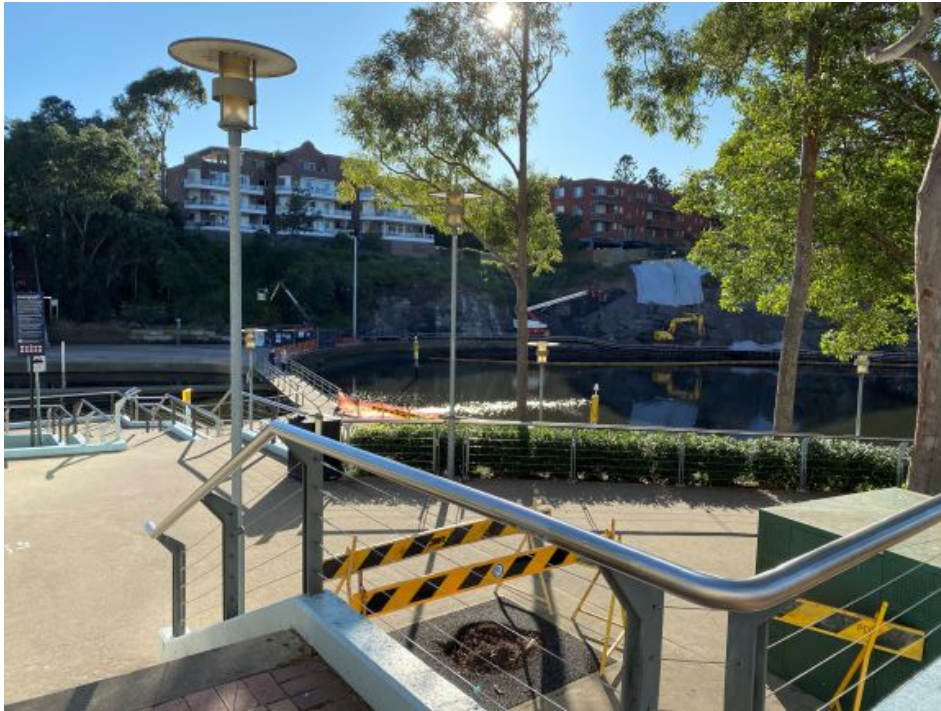
Photo 8: View north across river with Charles Street Weir in midground, Escarpment Boardwalk and Stewart Street Stairs under construction against the escarpment, and residential apartment buildings on top of the escarpment in the background
