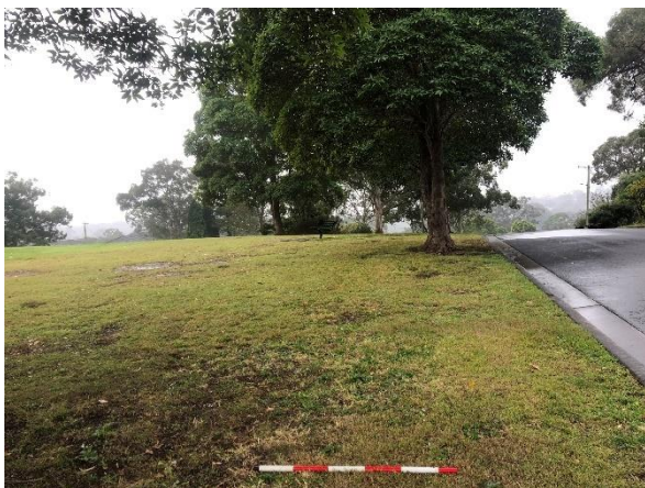
Figure 11: Slumping at location of the former Kishnaghur
