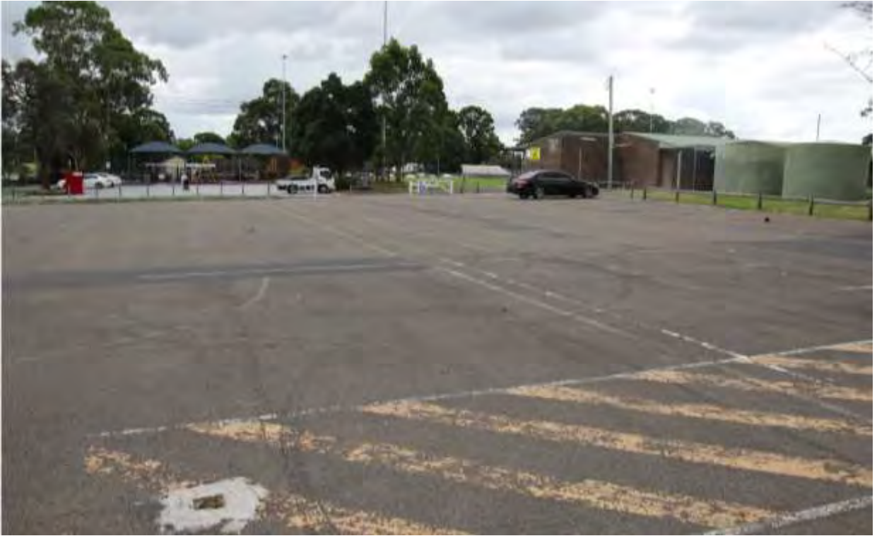
Photo 4.2: The southern off-street car park (79 parking spaces) (Photo: Traffic Engineering Centre Pty Ltd)
