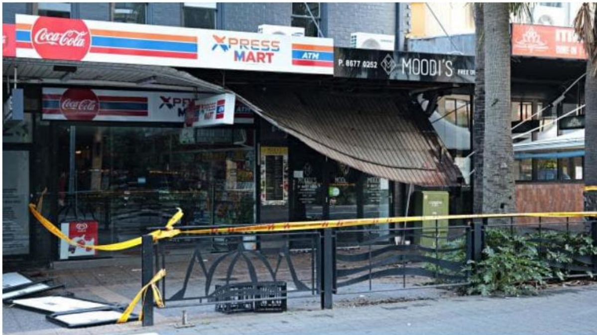
Damage caused by yesterday's massive storm on Church St Parramatta on the 9th of February 2019. Sydney was hit by a massive storm causing wide spread damage across Sydney. Picture: Adam Yip Source: News Corp Australia
