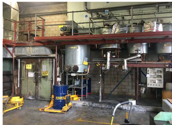
Photo 6 – Drum and AST storage area (McNeill Plastics).
