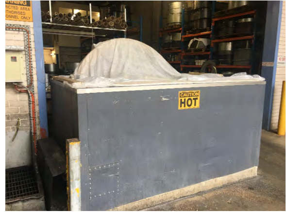
Photo 8- Conditioning tank (McNeill Plastics).
