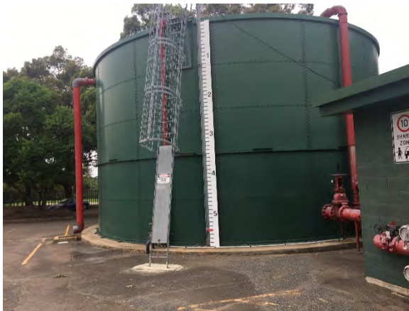
Photo 3. Fire water tank
