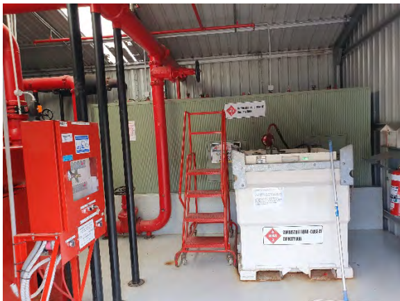
Photo 3. Diesel generator in fire pump room, located in the north west portion of the site.
