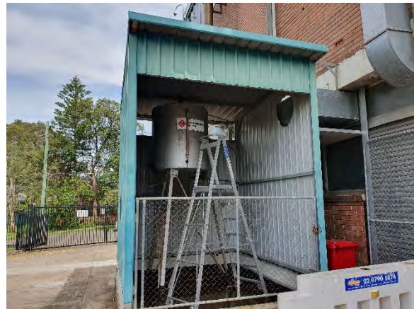
Photo 8. Diesel AST located in the southwest portion of the site.
