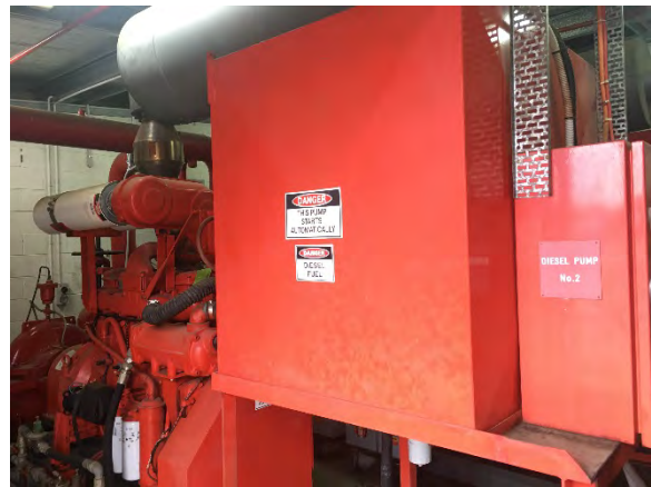
Photo 4. Diesel generator in fire pump room.
