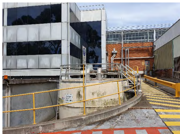
Photo 6. Enthalpy tank containing water.
